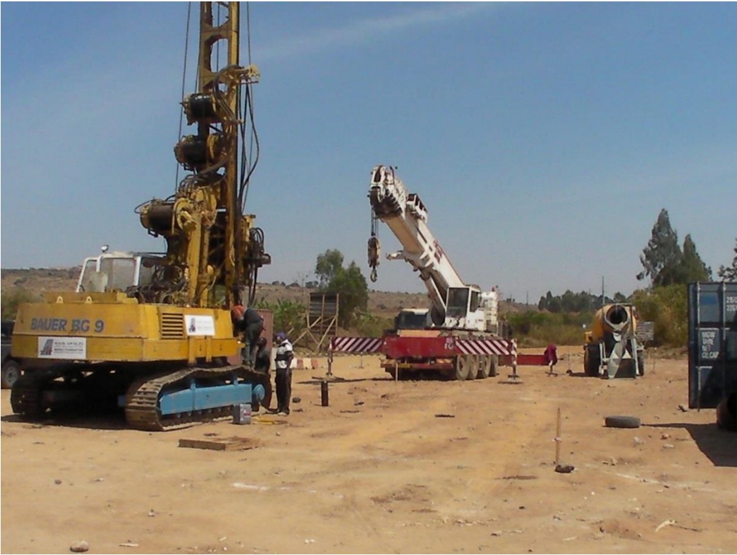
BG 9 Big Diameter Drilling Rig ( 109 Piles diam. 600 mm in Sumbawanga Leila Bridge, Tanzania)
