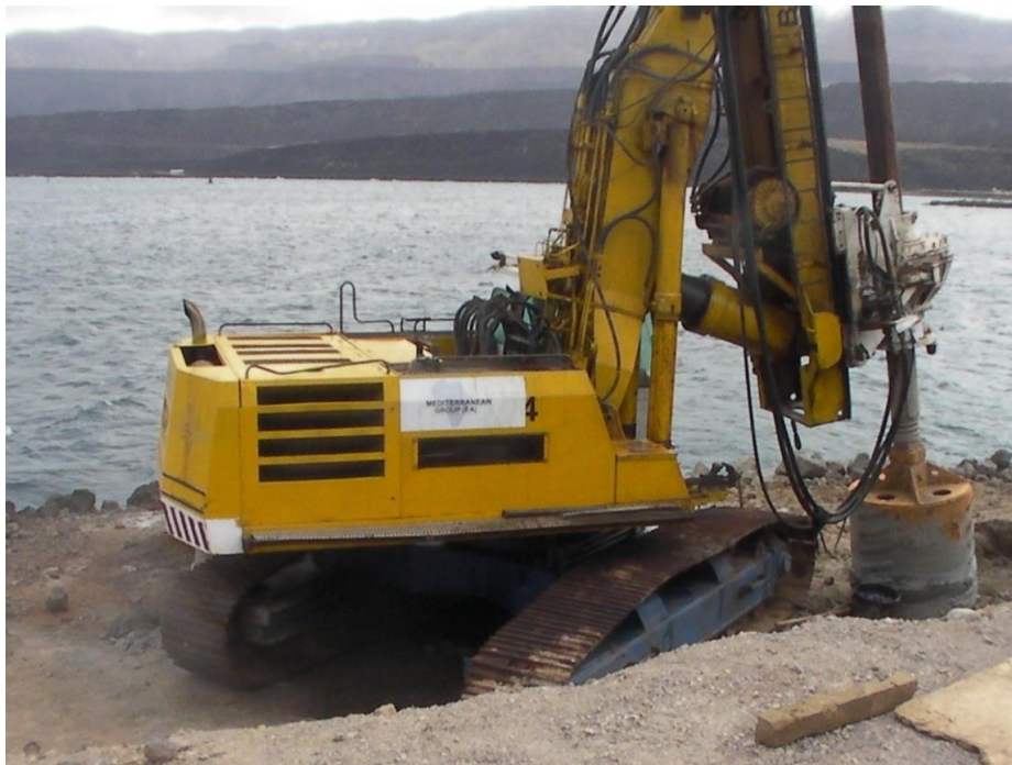
BG 14 Big Diameter Drilling Rig for Salt Exportation Port in Djibouti - ( 98 Off Shore Piles diameter 1200 mm drilled from barge, 9 Piles on Shore)
