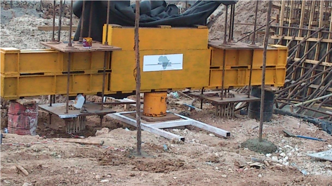
Pile Load Testing (up to 600tons at NHC Plot 300 Project, Dar Es Salaam Tanzania)
