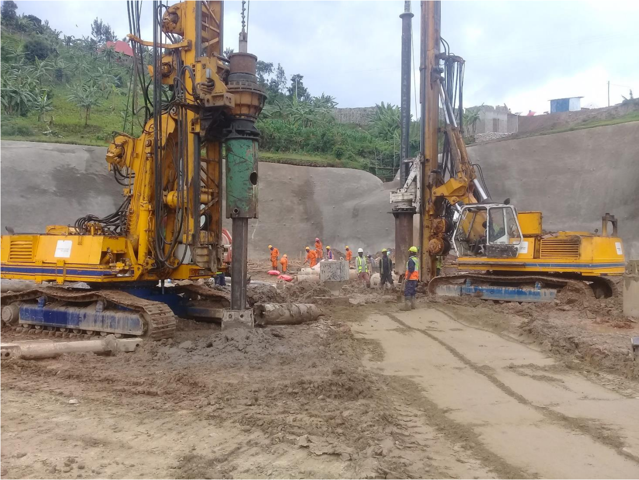
BG-9 and Delmag Drilling Rigs - SPLK Gas Power Plant Project- Lake Kivu, Rwanda
