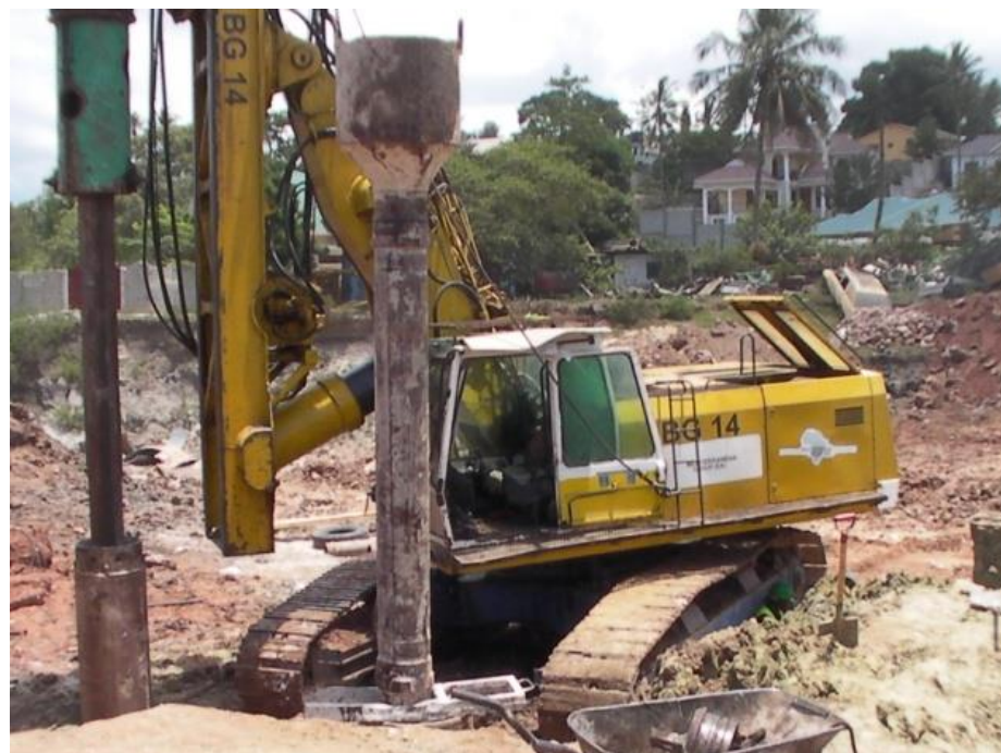
BG 14 Big Diameter Drilling Rig for Kinyerezi Bridge Dar Es Salaam, Tanzania - ( 68 Piles diameter 600 mm )
