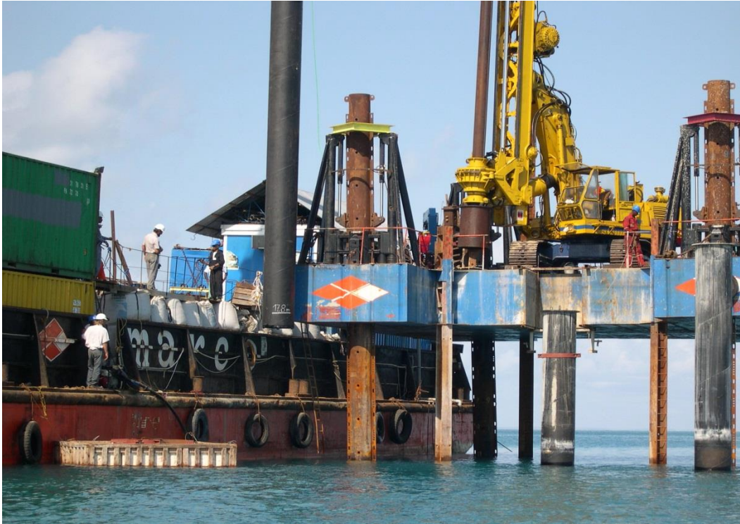
Big Diameter BG 11 Drilling Rig on Jack Up Pontoon (76 Piles diam. 1000 mm for Offshore Foundation Works Songo Songo, Tanzania )
