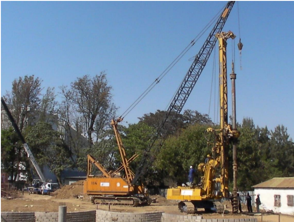
65 ton Crawler Crane and BG 9 Drilling Rig ( EAC Head Office in Arusha 262 Piles diam. 620 mm , 262 Integrity Test, 3 Load Tests )
