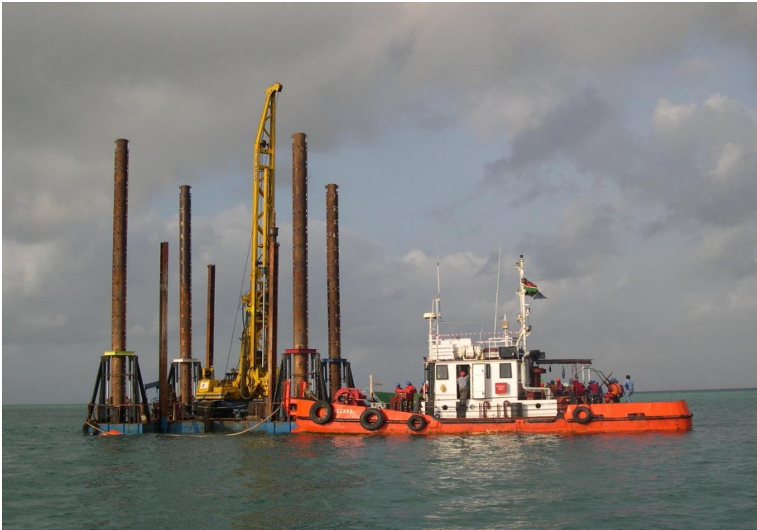
Big Diameter Drilling Rig on Offshore Jack Up Pontoon (For Offshore Foundation Works )
